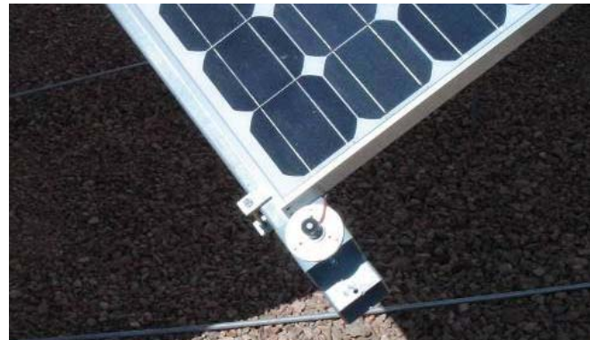
Fig. 6: Placement of the Pyranometer on the Tracker.
