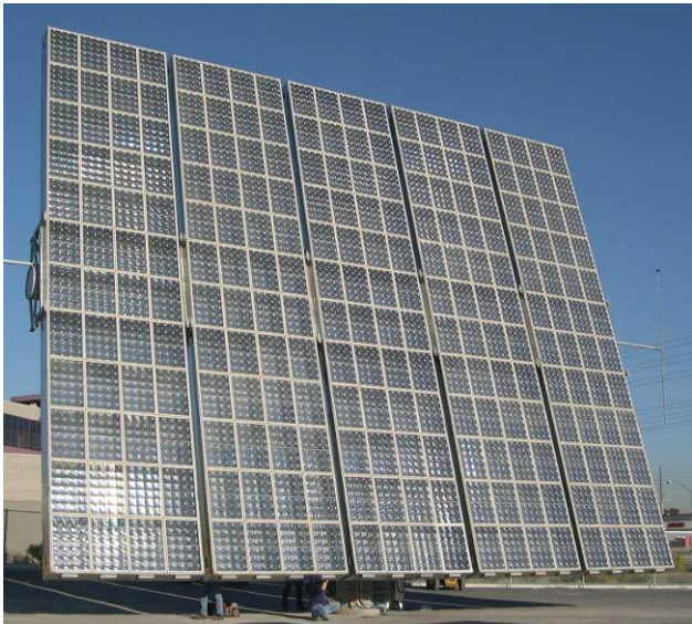
Figure 1-1. Amonix 25-kW system at UNLV.
