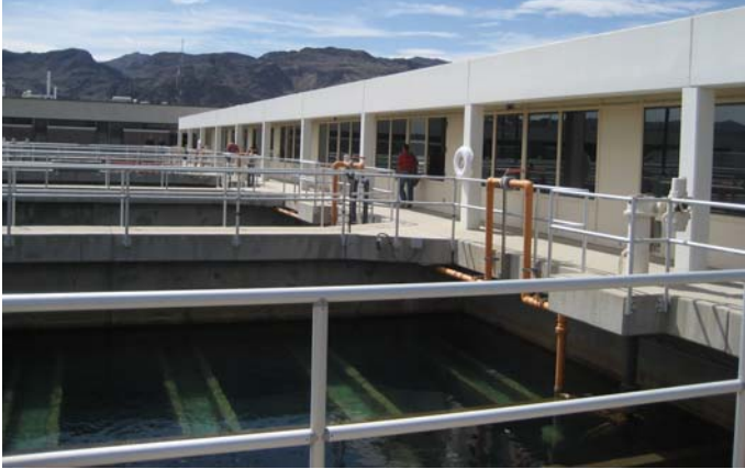
FIG. 4: FILTRATION TANKS AT THE PUMPING STATION.
