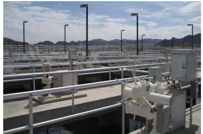
FIG. 3: FLOCCULATION BASIN AT THE PUMPING STATION.
