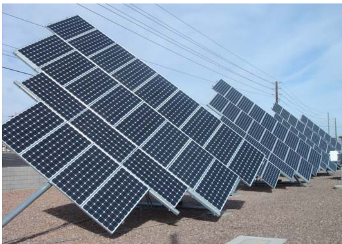
FIGURE 1: SOLAR PV ARRAY AT THE HYDROGEN FILLING STATION.
