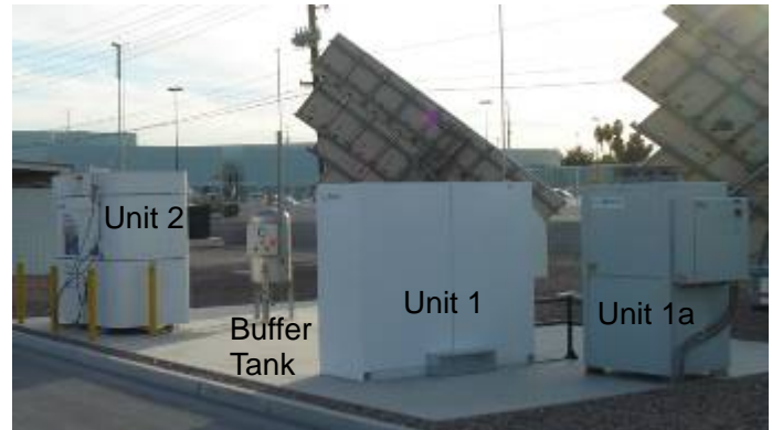
FIGURE 2: HFS GENERATION AND STORAGE EQUIPMENT.
