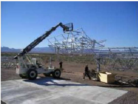
Figure 2. Installation of the Solar Collector Assemblies at the test site (Photo from Solargenix)
